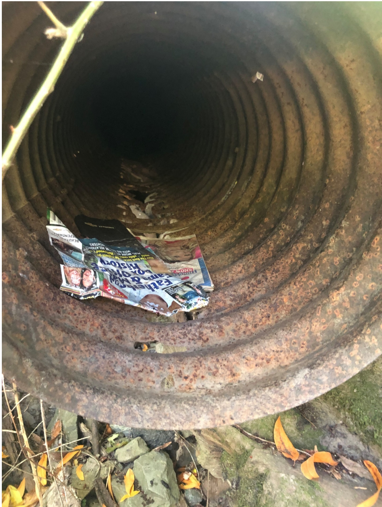
Figure 6. Culvert outlet rusted through at Map Point 1.
