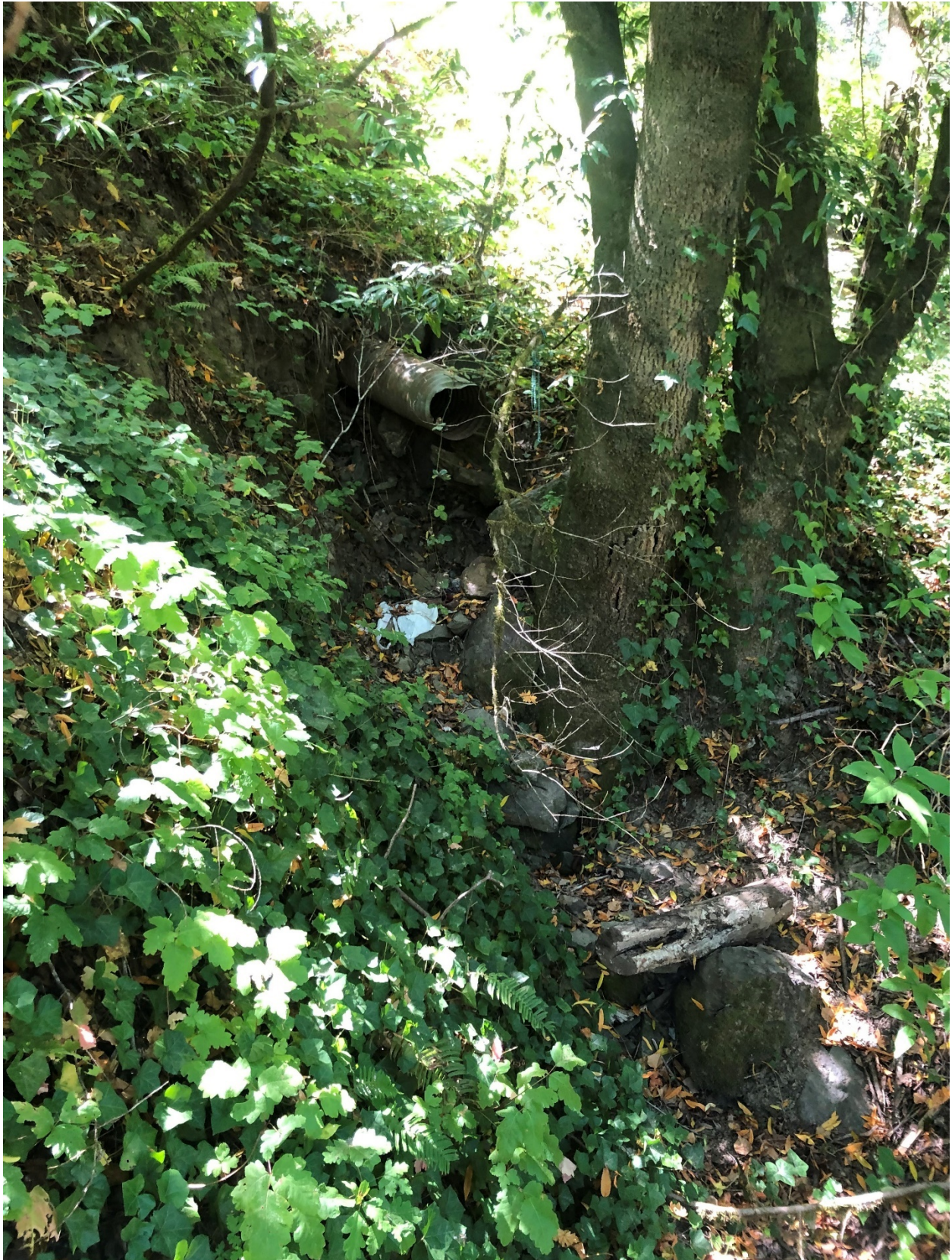
Figure 5. Shotgunned culvert outlet on Neeley Road at Map Point 1.
