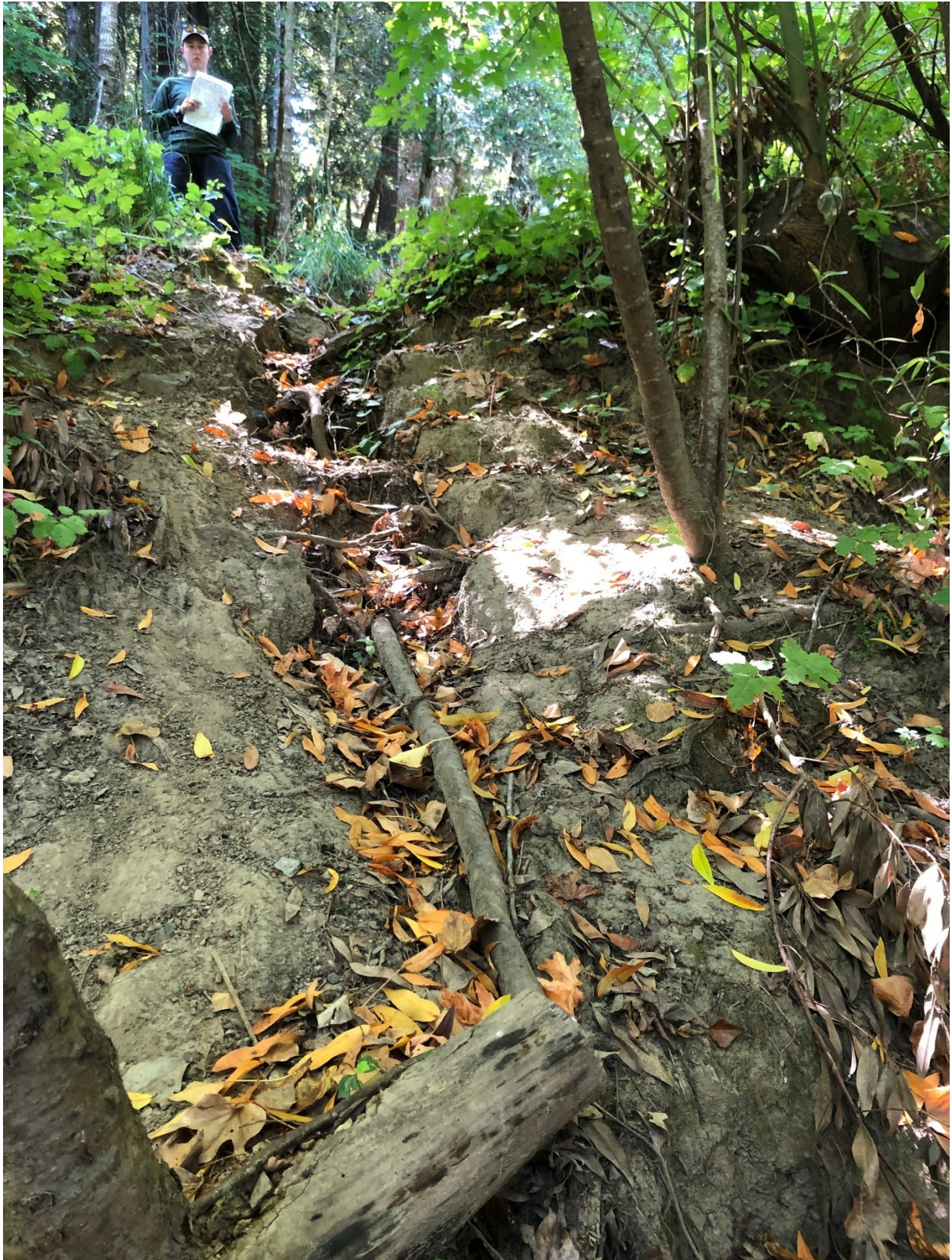
Figure 4. Erosion on outboard edge of Neeley Road at Map Point 1.
