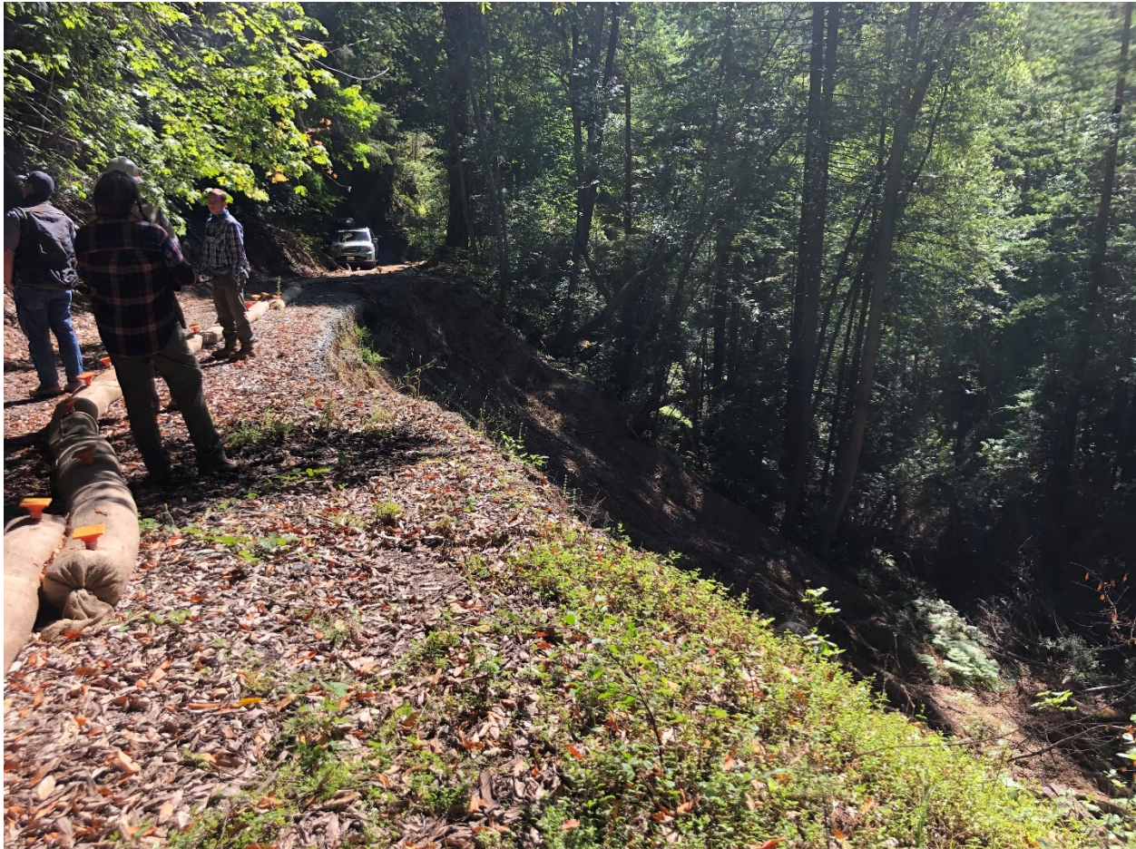
Figure 1. Looking northeast (downhill) and fill failure at Map Point E.
