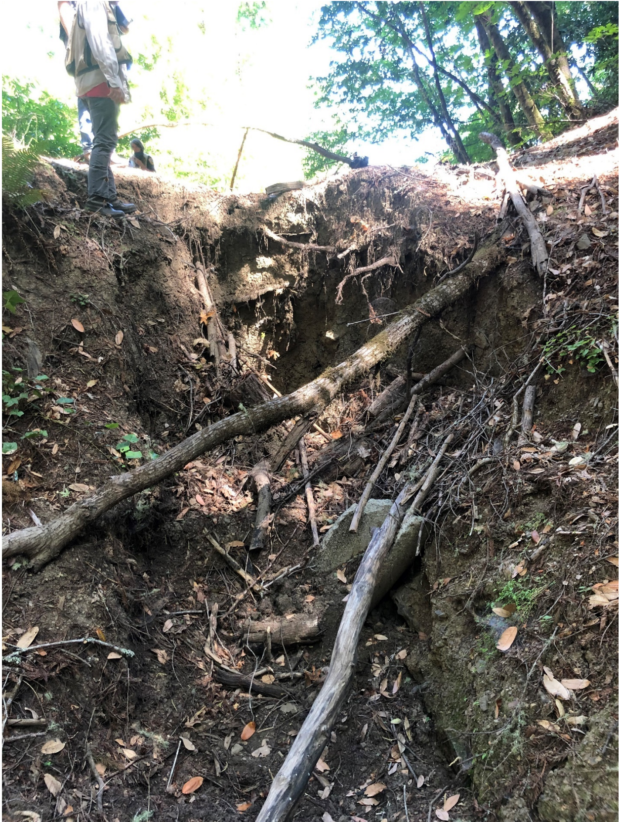
Figure 2. Inlet and over-steepened banks at inlet of culvert at Map Point 1.
